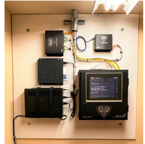
Information Technology assists Fire Rescue with the new enterprise Station Alerting infrastructure.
