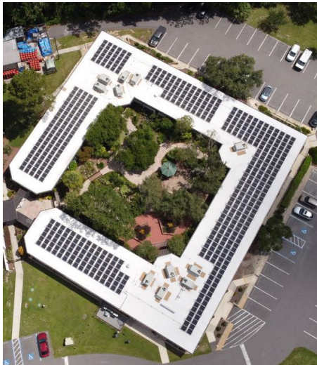
R3M installed a 122kW solar panel system on the roof of the Cooperative Extension Office for continued sustainability efforts.
