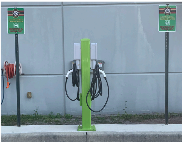
Fire Rescue provides EV charging stations.
